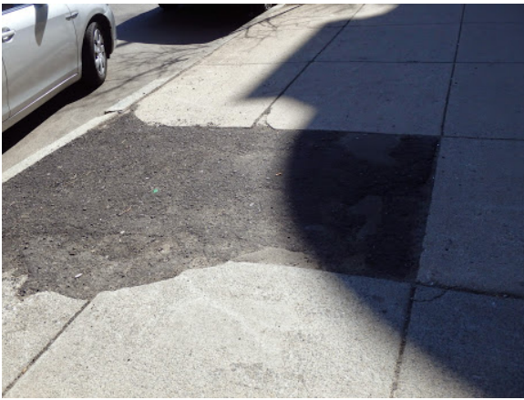
Asphalt Patch Westland Avenue south side
