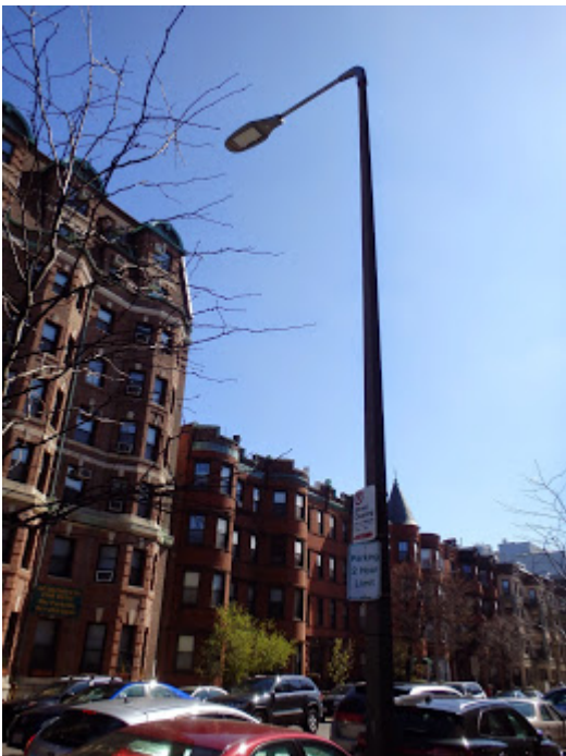
Light fixtures in street section without upgrade
