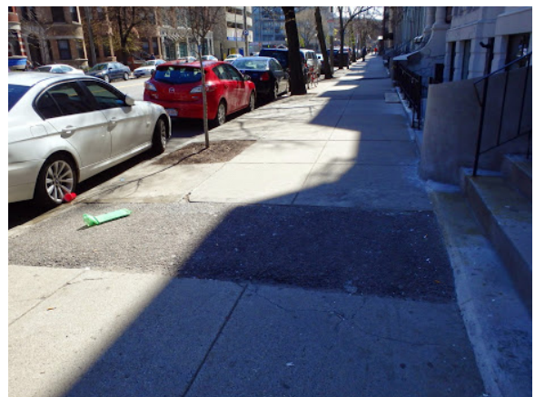
More asphalt patching south side Westland
