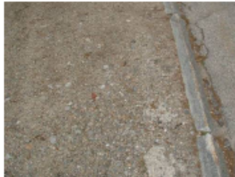
Figure 32 Gravel mix between sidewalk and curb at Agassiz Road bridge. (May 25, 2011)
