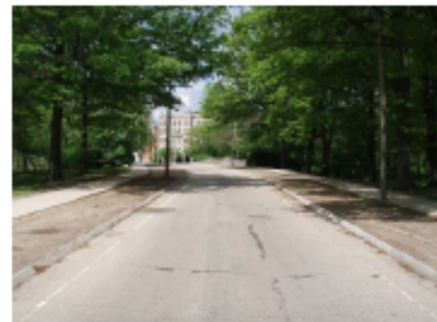
Figure 25 Agassiz Road, facing west towards bridge and Park Drive. (May 25, 2011)
