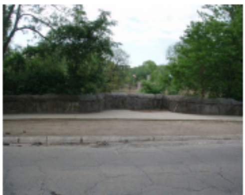
Figure 41 Overgrown vegetation along Agassiz Road Bridge (May 25, 2011)
